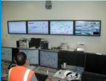
GWR Control Room
