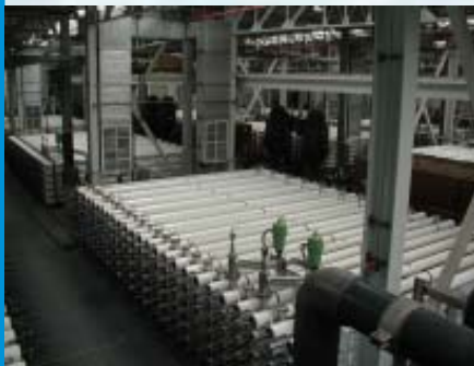
Reverse Osmosis Building
