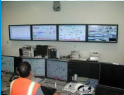
GWR Control Room
