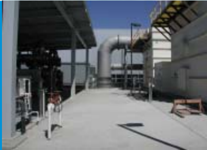
Decarbonator Feed Pipe
