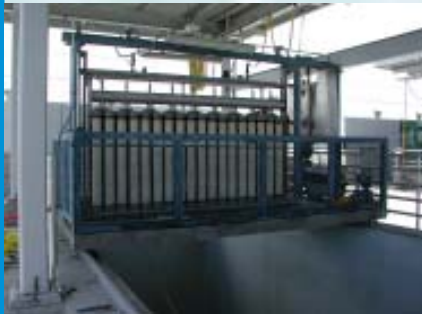
AWPF Microfiltration - Rack of Membrane in MEMSAP Unit
