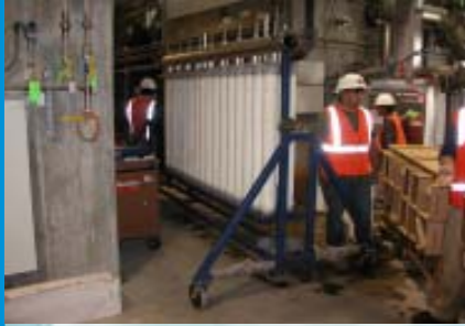
AWPF Microfiltration - Installed Membrane in a Rack
