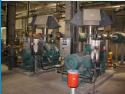
AWPF Microfiltration Blowers
