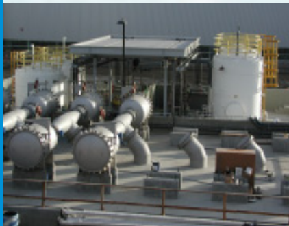
AWPF Cartridge Filters/Chemical Tankage (Caustic Soda & Citric Acid)
