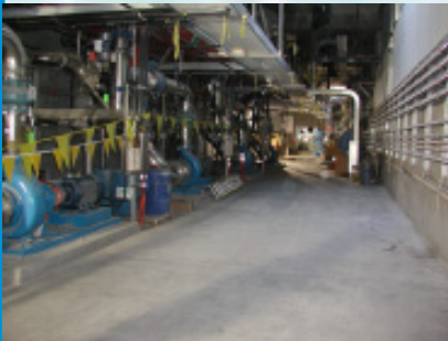
AWPF Microfiltration Gallery Piping
