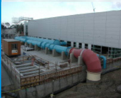
AWPF Microfiltration Break Tank/Reverse Osmosis Transfer Pump Station
