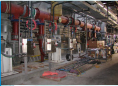
AWPF Microfiltration Waste Backwash Pump Station
