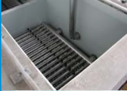
AWPF Microfiltration Cell
