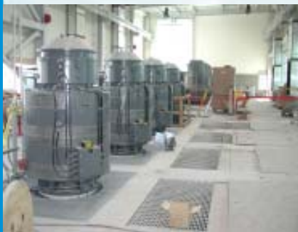
AWPF Product Water Pump Station
