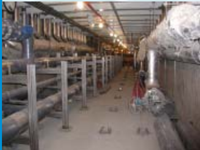
AWPF Reverse Osmosis Pipe Gallery
