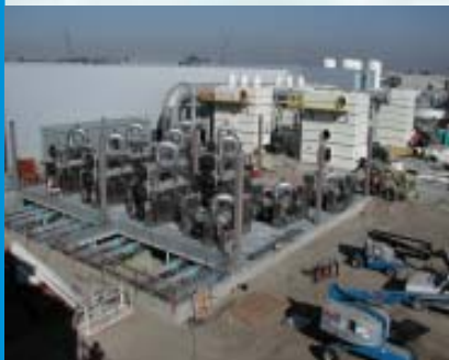
AWPF Ultraviolet Light (Foreground) Decarbonators (Background)
