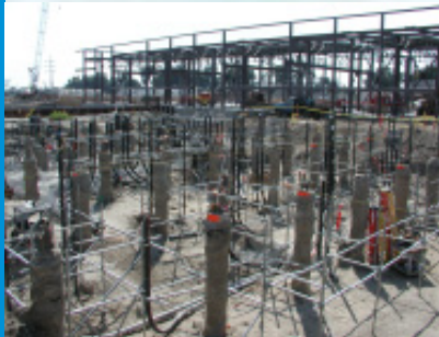
AWPF Reverse Osmosis Electrical Building Underground Conduit
