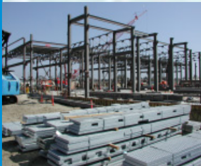
AWPF Reverse Osmosis Structural Steel Framing
